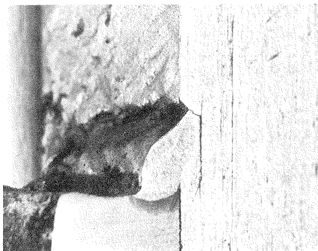
FIGURE 12 Crack growth in span F hanger.
