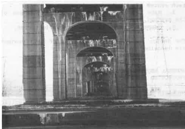
FIGURE 1 Salt staining on pier bents, Burlington Bay Skyway.
