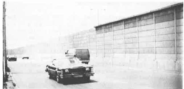
FIGURE 3 View from the residential side showing T-top and conventional barriers.
