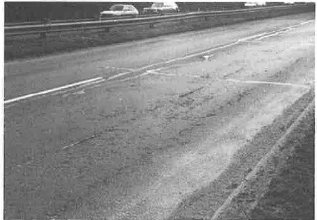
FIGURE 10 Surface deterioration and raveling on HMAC overlay, Merritt Parkway.
