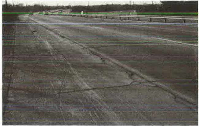
FIGURE 13 Severe faulting in outside lanes of PCC pavement along I-95, Housatonic River Bridge.
