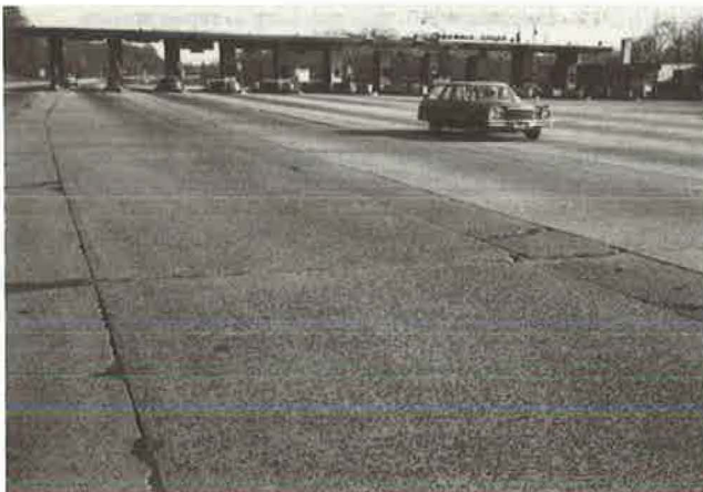
FIGURE 12 Structural condition of PCC pavement along I-95, Norwalk toll station.
