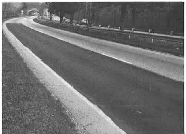
FIGURE 11 Full lane width skin patching to repair surface deterioration along Merritt Parkway.
