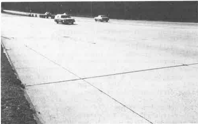
FIGURE 9 Structural condition of PCC pavement on Merritt Parkway at Greenwich toll station.
