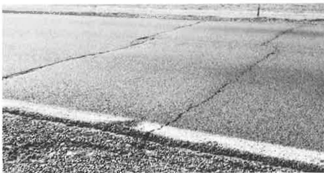
FIGURE 3 Heave of material above underlying hot-mix patch.
