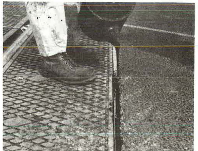
FIGURE 12 Hot-poured rubberized sealant has performed best.
