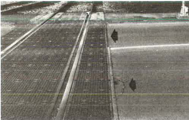
FIGURE 2 Failure to seal joint resulted in pavement cracking. Note that one-half is sealed but has no header board and is performing better.
