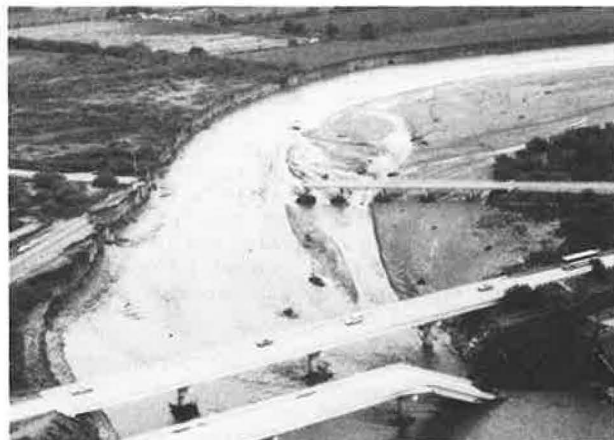
FIGURE 6 Oblique aerial downstream at two bridges destroyed by bank scour immediately below Martinez Hill.
