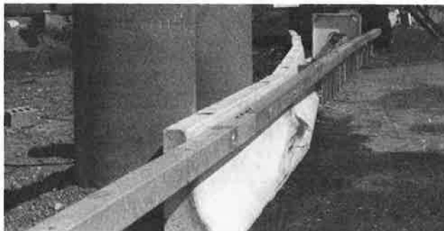
FIGURE 2 Pier-protection barrier for Tests 76 and 77: extending the box beam across Section A.
