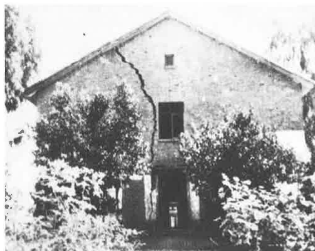
FIGURE 3 Crack on gable of building near jarrah.
