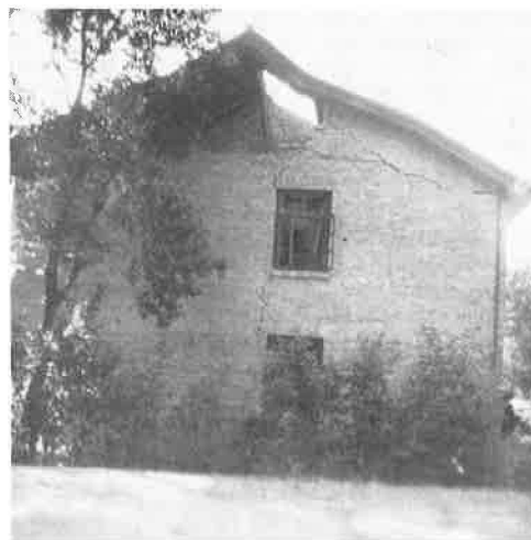
FIGURE 5 Collapse of roof.
