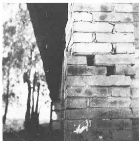
FIGURE 2 Horizontal displacement of corridor brick pillar.
