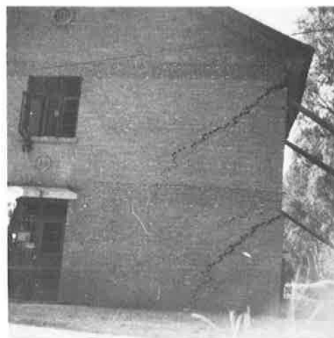
FIGURE 4 Inclination of external wall.
