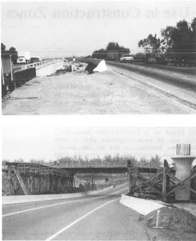
FIGURE 1 Typical use of precast concrete safety shape barriers in work zones: top, bridge widening project; bottom, construction overpass.
