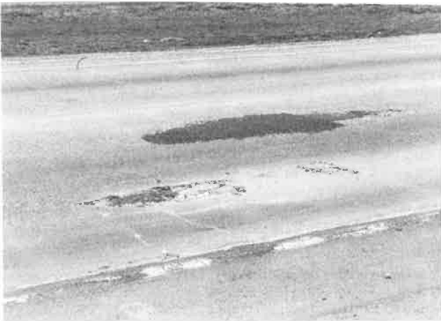
FIGURE 1 Deterioration of CRCP.
