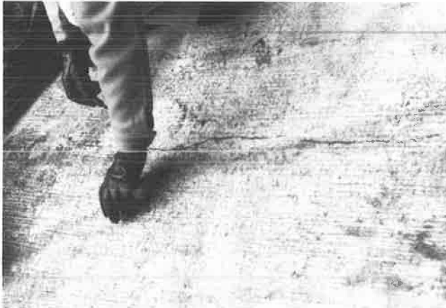
FIGURE 7 Photograph of deck crack marked and observed during LP6.
