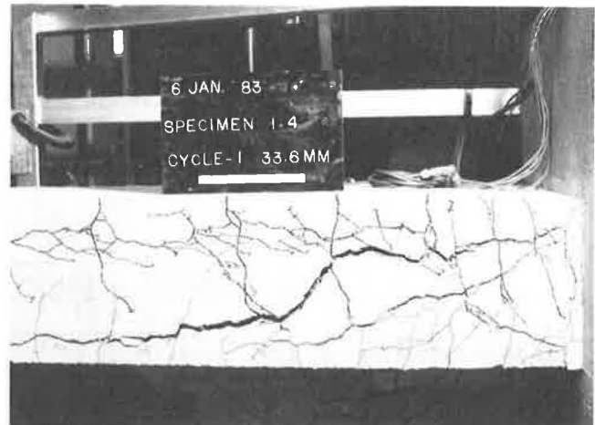
FIGURE 10 Final crack pattern for Specimen 1-4, 4δy/l.
