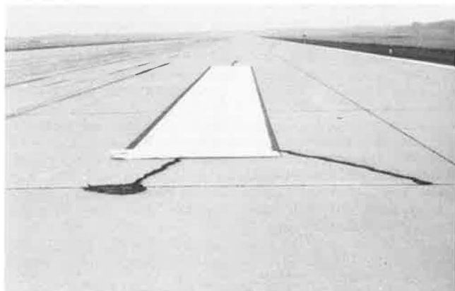
FIGURE 2 Paint stripe cracking caused by pavement curl.
