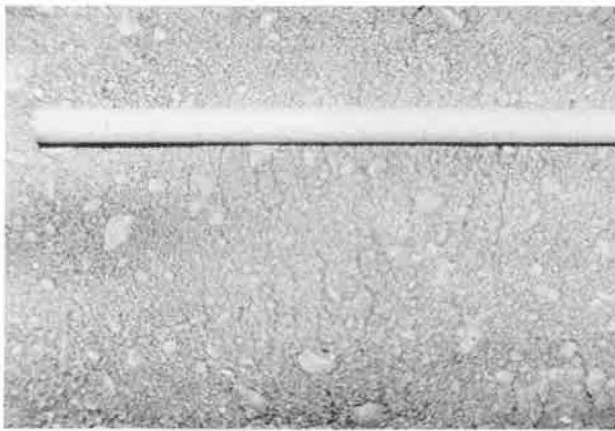
FIGURE 16 Simulated construction cracks.
