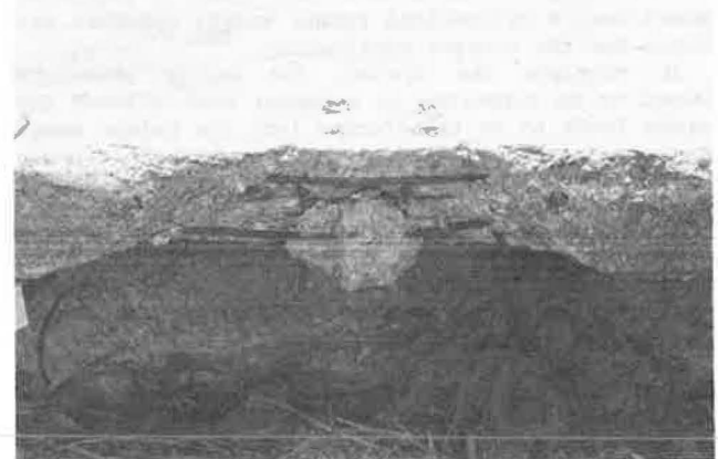
FIGURE 5 Example of worst bridge deck damage before testing.
