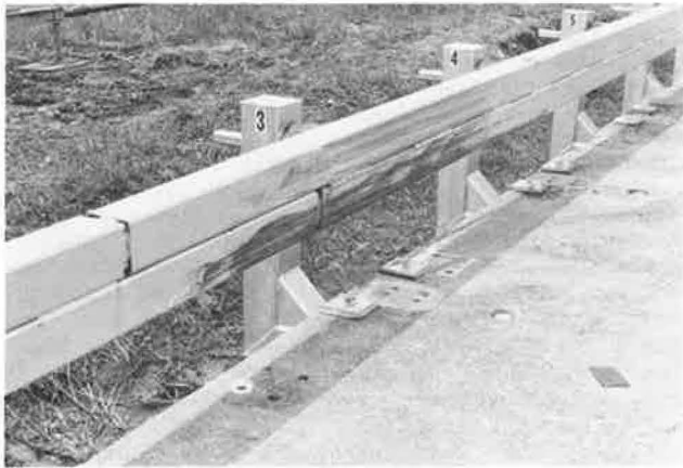
FIGURE 7 Bridge rail after Test 1.
