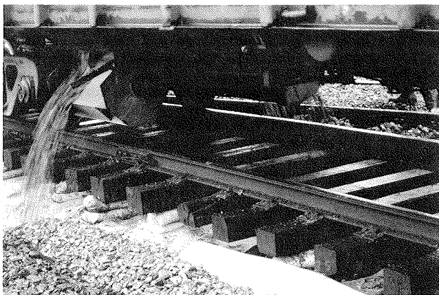
FIGURE 16 Filling French drain of turnout with ballast showing track supported by ballast bags.
