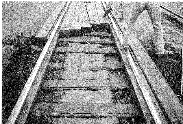
FIGURE 11 Typical condition of fouled grade crossing having inadequate drainage at centerline.
