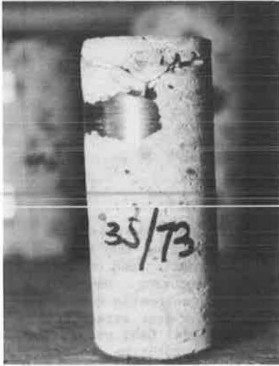
FIGURE 1 Corrosion-induced delamination in a concrete core.
