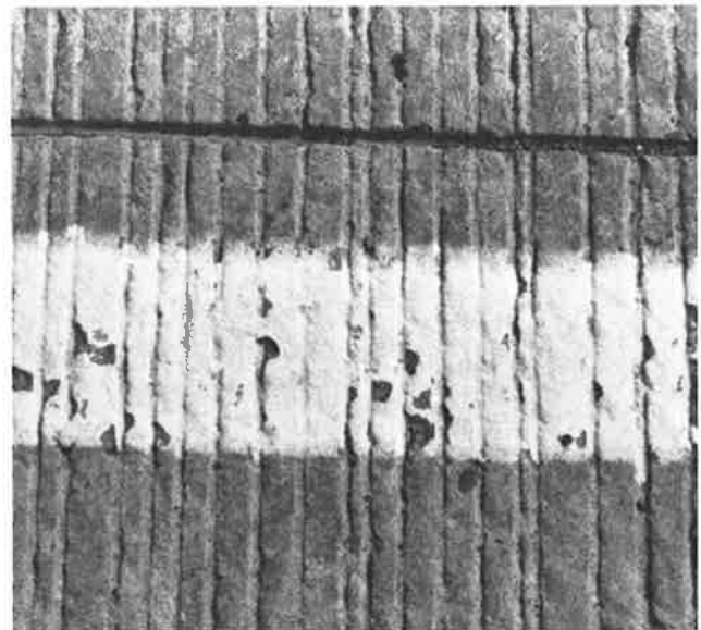
FIGURE 3 Loss of epoxy striping caused by chipping of peaks on fine-textured concrete pavement.
