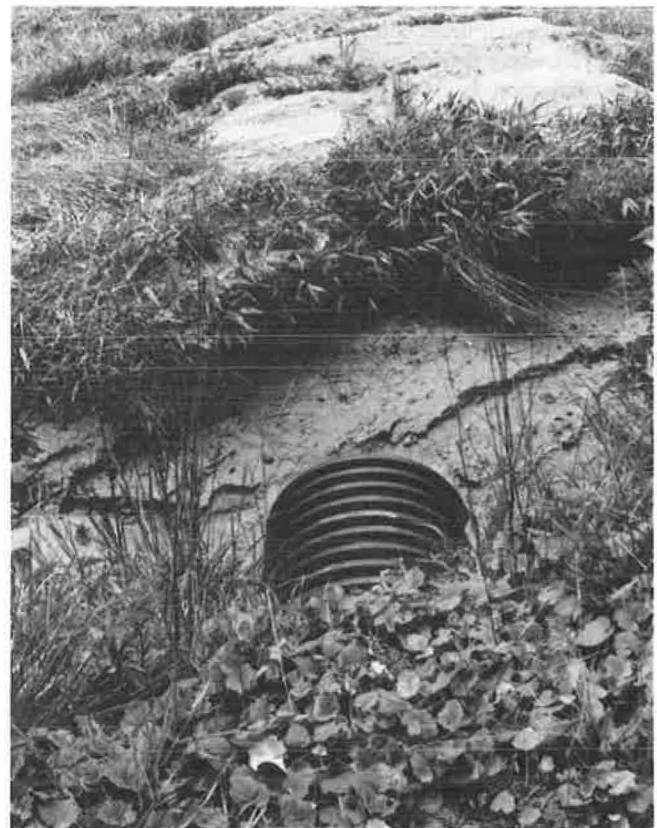
FIGURE 8 Outlet channel debris at NOB-145-3.58 indicative of force of storm flow.
