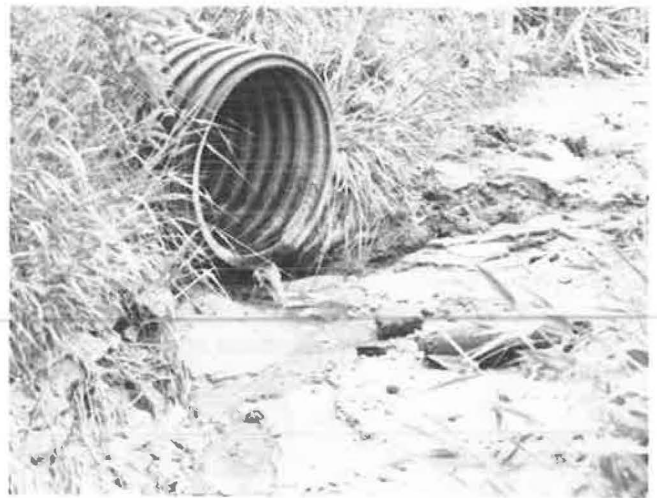
FIGURE 7 24-in. corrugated polyethylene pipe culvert at NOB-145-3.58: low pH and severely abrasive flow.
