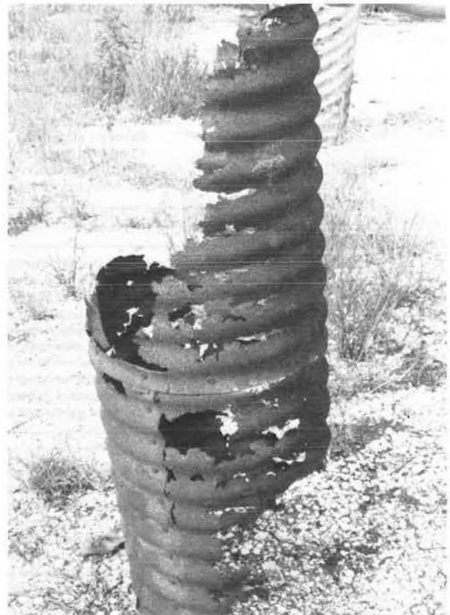
FIGURE 4 16-gauge galvanized steel after 10 years of exposure at Site 7.
