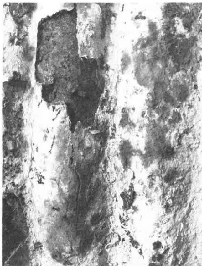
FIGURE 6 Corrosion between asbestos and base metal—Site 10.
