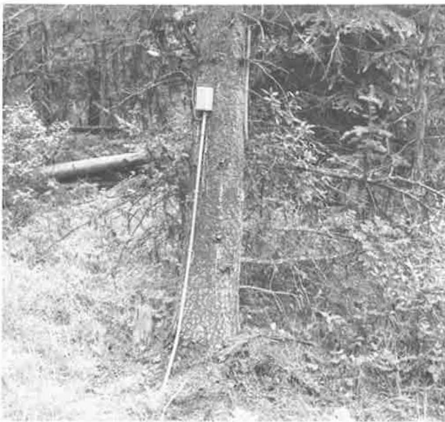
FIGURE 7 Junction box, Site D2-92-38.0; note air probe on branch slightly above and left of junction box.
