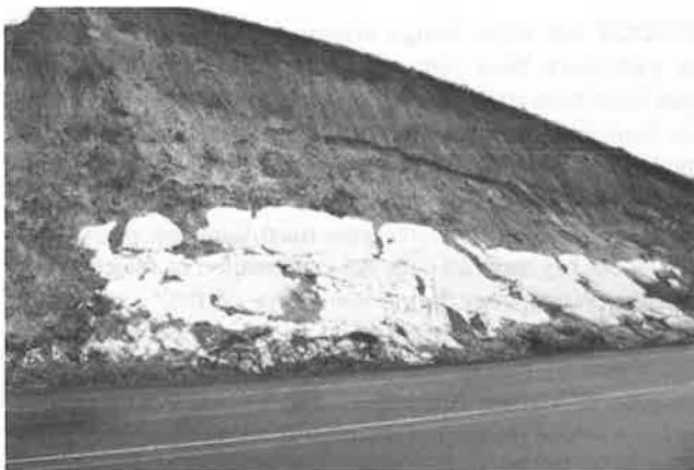
FIGURE 15 Shallow failure of road cut in loessial soils under melting snowdrift.
