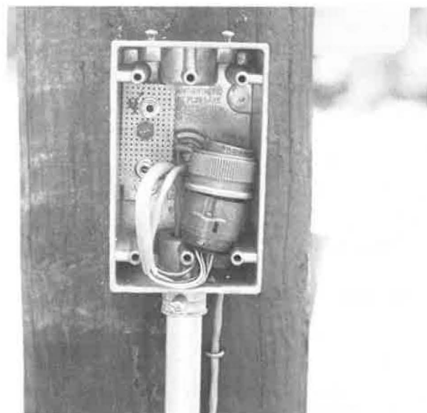
FIGURE 8 Ten-pin electrical connector at instrument string terminus and phono jacks for reading the 4- and 5-ft sensors, Site D2-92-23.95.
