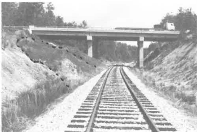
FIGURE 2 Railroad Underpass/US-64 slope failure.
