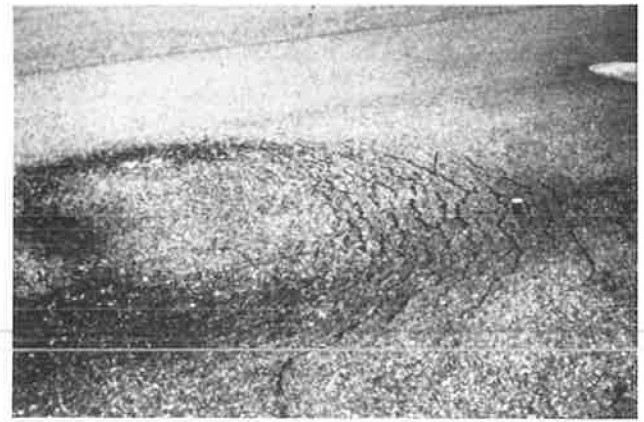
FIGURE 18 Typical crescent-shaped slippage cracks.
