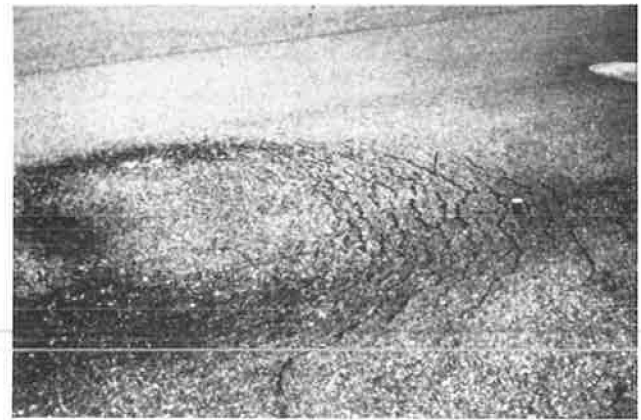
FIGURE 18 Typical crescent-shaped slippage cracks.
