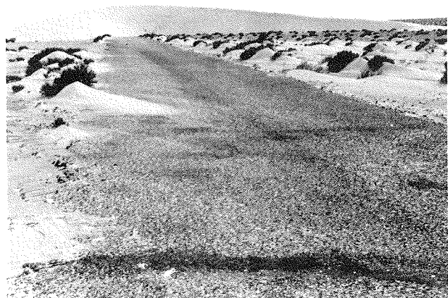
FIGURE 1 A migrating barchan has cut off the road from Laayoune to Bojador, 31.5 km from Laayoune.
