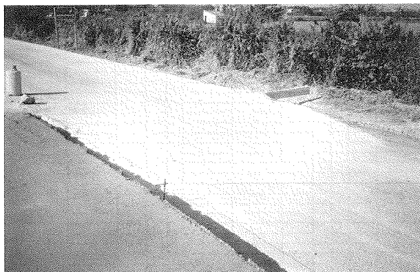
FIGURE 10 Sand wedge at construction joint.
