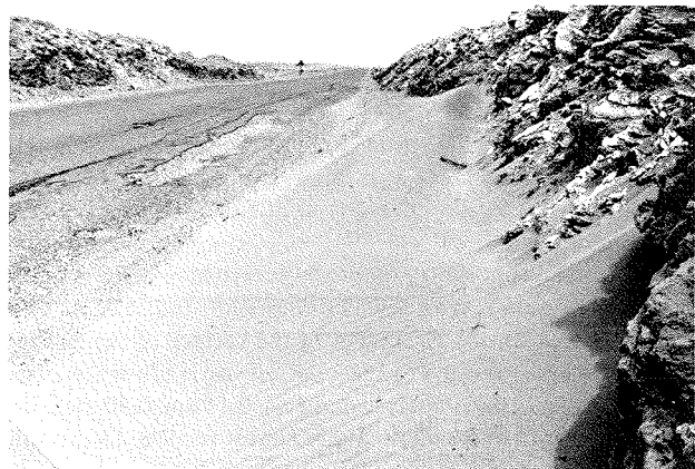
FIGURE 3 Cut section invaded by sand on the road from Tan-Tan to Laayaoune, 150 km to the south of Tan-Tan.
