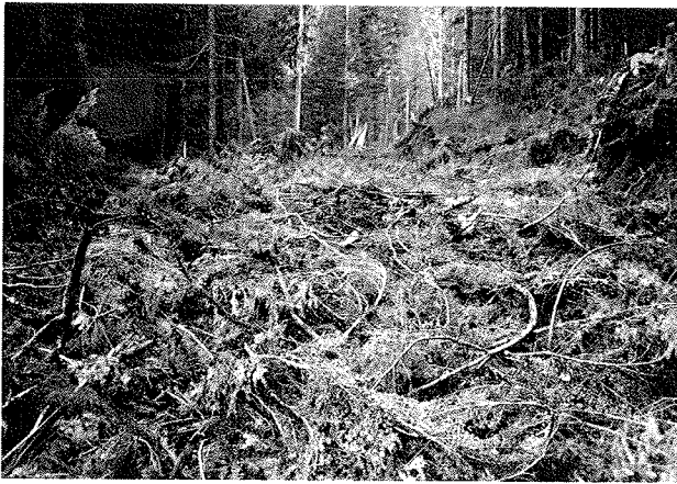
FIGURE 6 Timber slash placed on the road subgrade as corduroy before placing rock embankment in a terrain other than muskeg.
