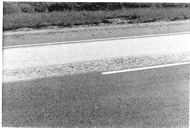
FIGURE 8 Bituminous pavement showing alligator cracking.
