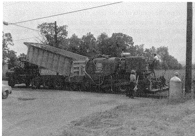
FIGURE 4 Recycled asphalt pavement being discharged into the Midland Motopaver on the Chester County project.
