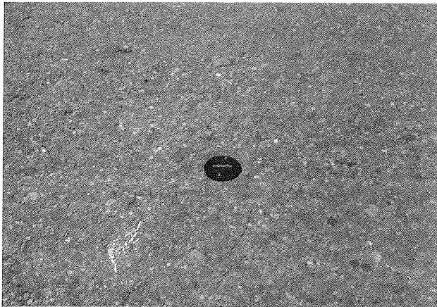
FIGURE 12 Large stones of recycled base showing through a single seal coat.
