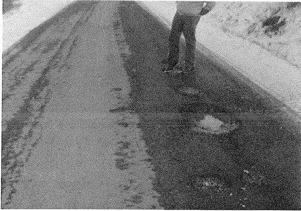
FIGURE 11 Roadway with potholes after the first winter on the Susquehanna County project.
