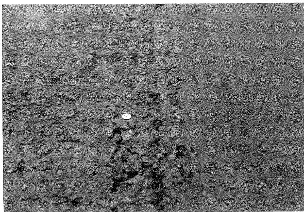
FIGURE 19 Roadway on the Luzerne County project; (l) without seal coat, (r) with seal coat.
