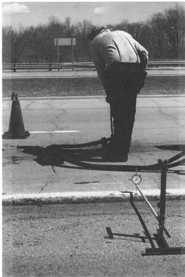
FIGURE 3 Deflection gauge in use during undersealing of a section of CRC pavement.
