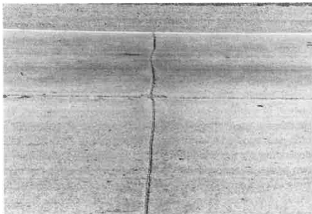
FIGURE 3 Typical crooked transverse joint.
