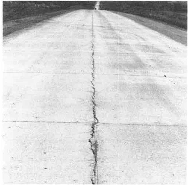
FIGURE 7 Typical random centerline cracking.
