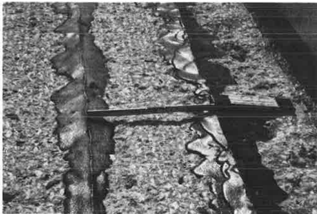
FIGURE 16 Placement of anode backfill material in the mound configuration is difficult because of the low viscosity of the material.
