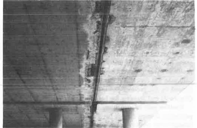
FIGURE 11 Deterioration of underside of deck because of water and salt intrusion under surface-mounted angle iron and preformed elastomeric joint assemblies.
