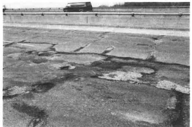
FIGURE 4 Continued deterioration of cracking shown in Figure 3 resulted in spalling of wearing surface to the interface with coke breeze asphaltic mixture.
