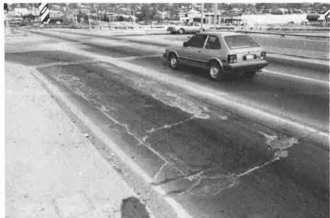
FIGURE 15 Deterioration of asphaltic concrete overlay caused by stopping of vehicles.
