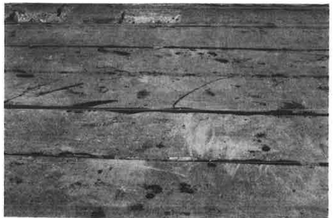
FIGURE 17 Improper placement of epoxy in slots to prevent shorts to high rebars.
