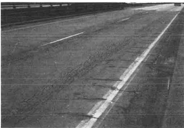
FIGURE 2 Longitudinal cracking in wheel paths of driving lane and transverse cracking in outer shoulder where coke breeze asphaltic mixture is being shoved from the wheel path.
