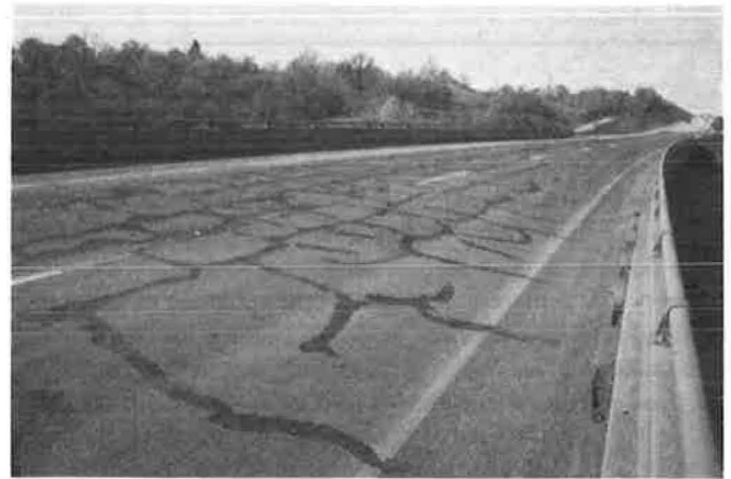
FIGURE 3 Cracking in wearing surface, porphyry asphaltic concrete, after first winter of exposure and frost heave.
