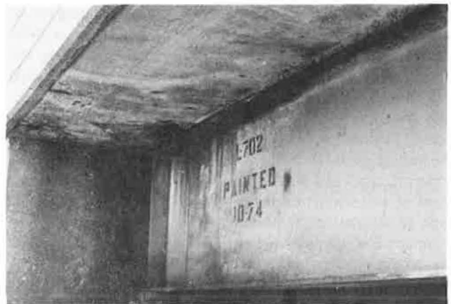
FIGURE 8 Corrosion product and water drained from deck through improperly placed drains caused staining and corrosion of steel stringers.
