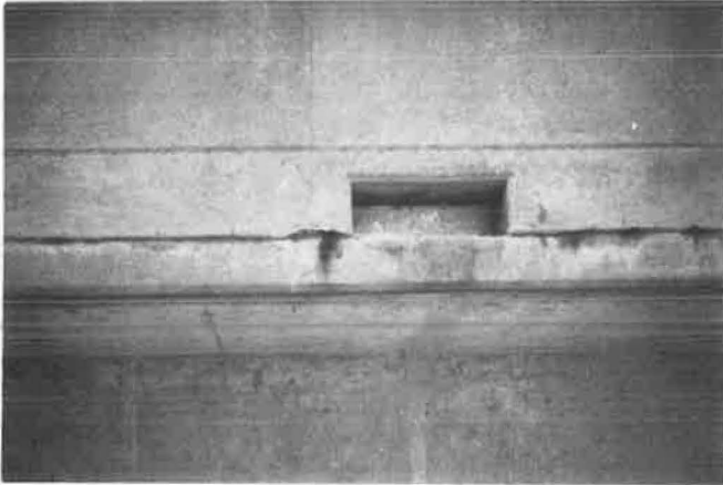
FIGURE 9 Deterioration continues in unprotected outer parapet areas. Curb outlet Number 3 during installation of cathodic protection in 1975.
