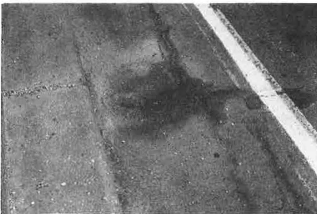
FIGURE 5 Corrosion of anodes caused swelling of asphaltic layers, cracking, and emission of brownish-colored corrosion product on surface.
