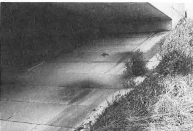
FIGURE 6 Corrosion product from anodes migrated to curb outlets provided for water drainage, causing staining on slope protection and bridge parapet walls.
