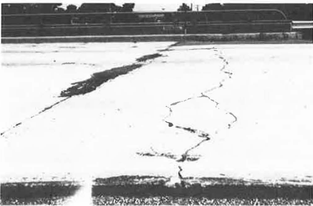
FIGURE 4 Approach slab distress.
