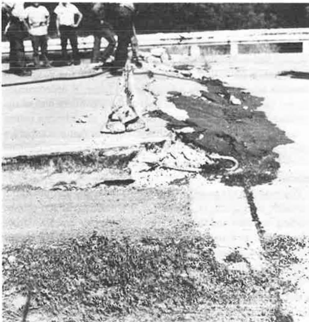
FIGURE 6 Approach slab blowup.
