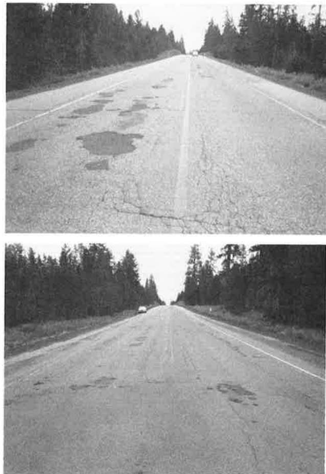
FIGURE 3 Typical pavement condition before overlay: (top) milepost 158.21 looking south and (bottom) milepost 158.26 looking north.
