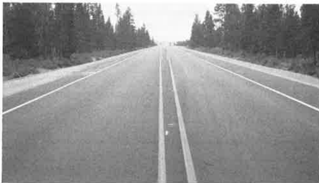
FIGURE 7 Typical pavement condition of Class-C mix with polymer-modified asphalt and lime-treated aggregate (milepost 161.46 looking south).
