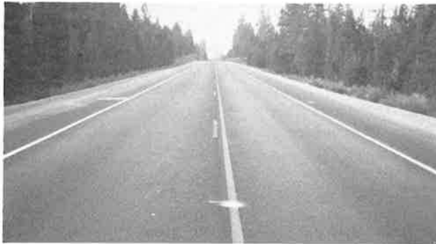
FIGURE 5 Typical pavement condition of PlusRide after overlay (milepost 158.21 looking south).
