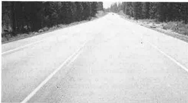
FIGURE 6 Typical pavement condition of Arm-R-Shield after overlay (milepost 158.62 looking south).
