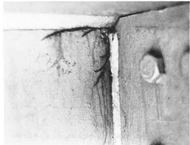
FIGURE 1 Typical cracks in web at floor beam-to-girder connection.
