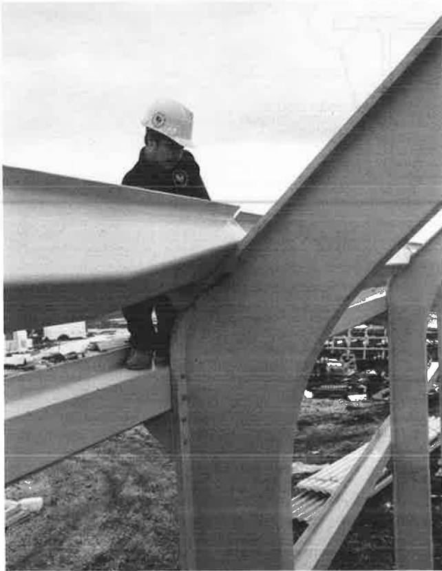
FIGURE 5 Deep rigid-frame knee without splice or connections reduces stress levels and eliminates problem of fasteners at high-moment corner.
