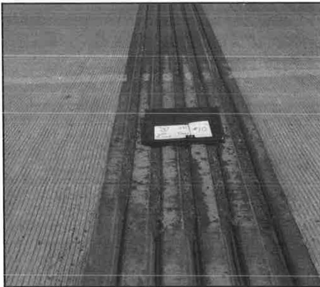
FIGURE 16 A modular joint showing debris accumulation.
