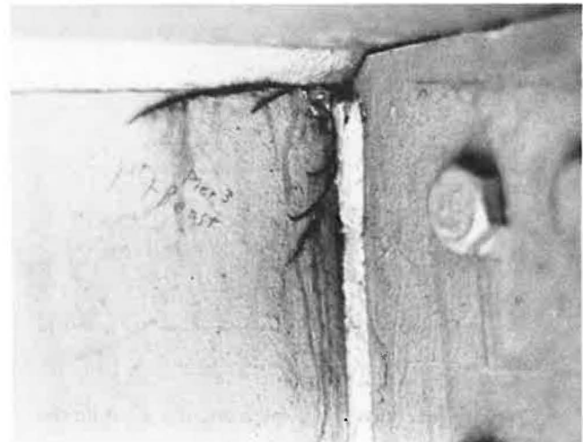
FIGURE 1 Typical cracks in web at floor beam-to-girder connection.
