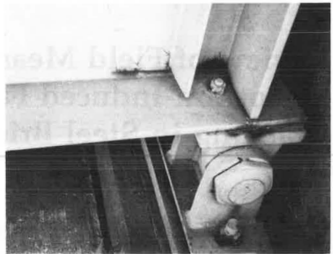
FIGURE 4 Cracking at base of bearing stiffener and adjacent transverse stiffener.
