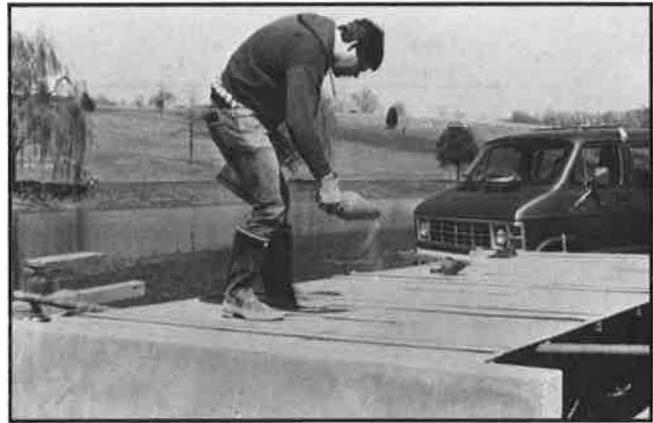
FIGURE 4 Sand aggregate applied to polyester resin to form polymer concrete wearing course.
