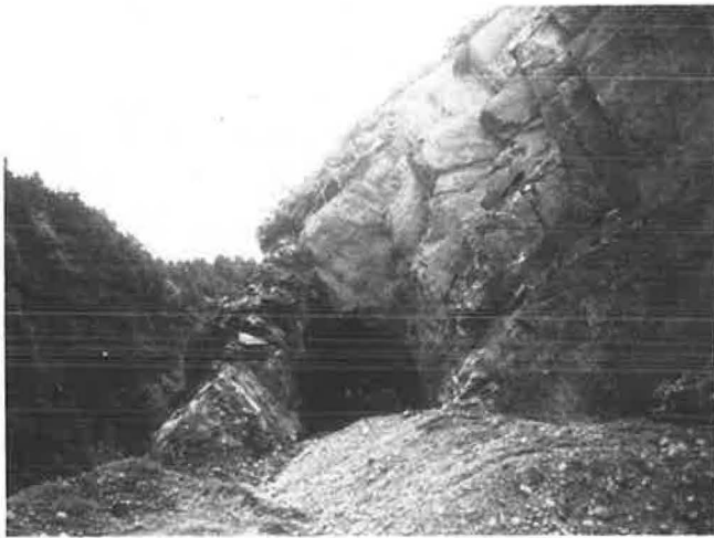
FIGURE 5 North portal showing tension crack and track protection.
