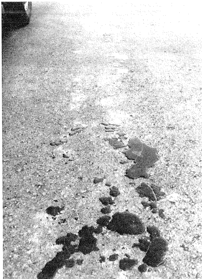
FIGURE 5 Patches of water emerged from pavement in hot afternoon and left stains behind when evaporated.
