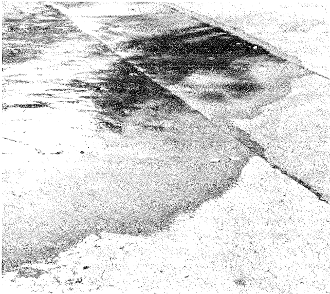
FIGURE 8 Water-induced cracks in pavement before formation of pothole.
