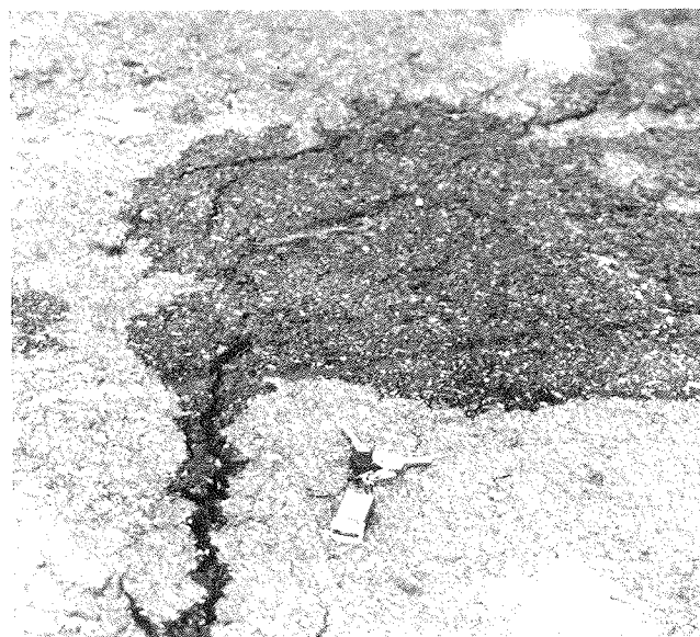
FIGURE 7 Outflow of water and fines from curb joint.
