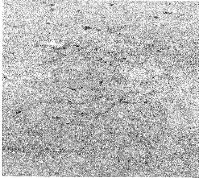
FIGURE 9 Water bleeding from utility trench joint; photo taken 9 hr after rain had stopped.
