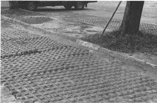
FIGURE 4 Studded-slab pavement damage by tree-root heaving.
