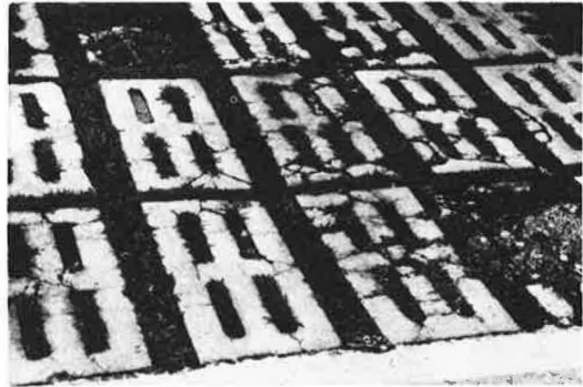
FIGURE 7 Cracked precast perforated slabs.
