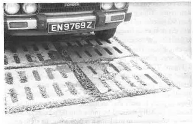
FIGURE 10 Rocking and cracked Type B perforated slabs.
