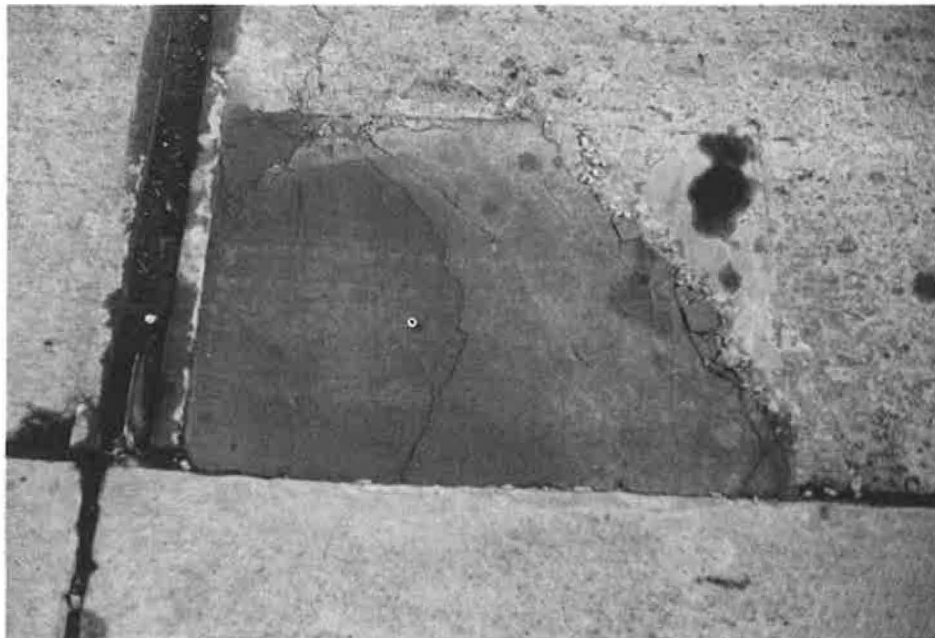
FIGURE 11 Example of failed patch at corner break.
