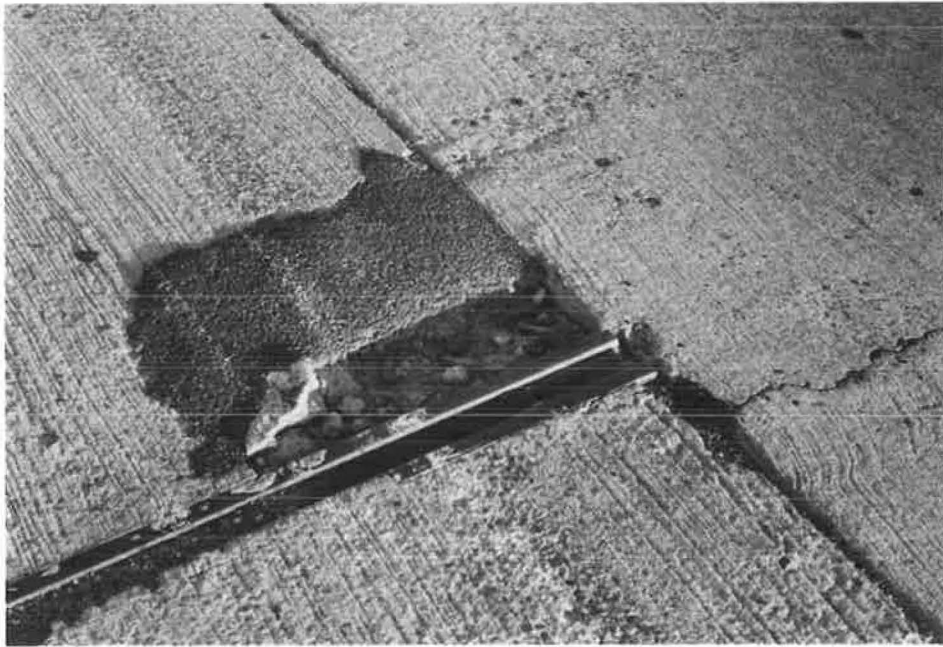
FIGURE 12 Failed asphalt patch at corner break.
