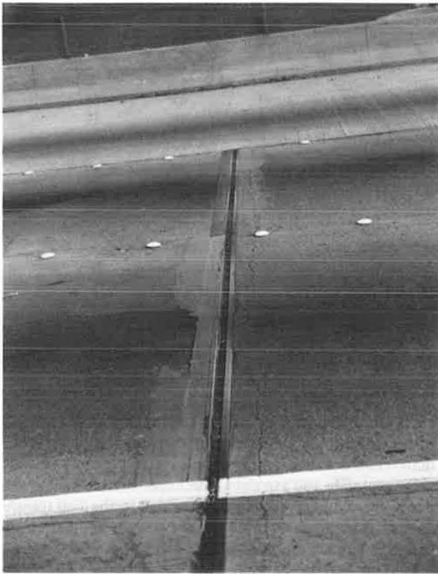
FIGURE 6 Epoxy patch and transverse crack at a joint.
