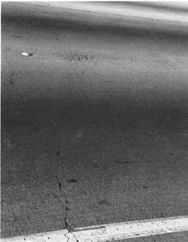
FIGURE 15 Spalling of transverse crack.
