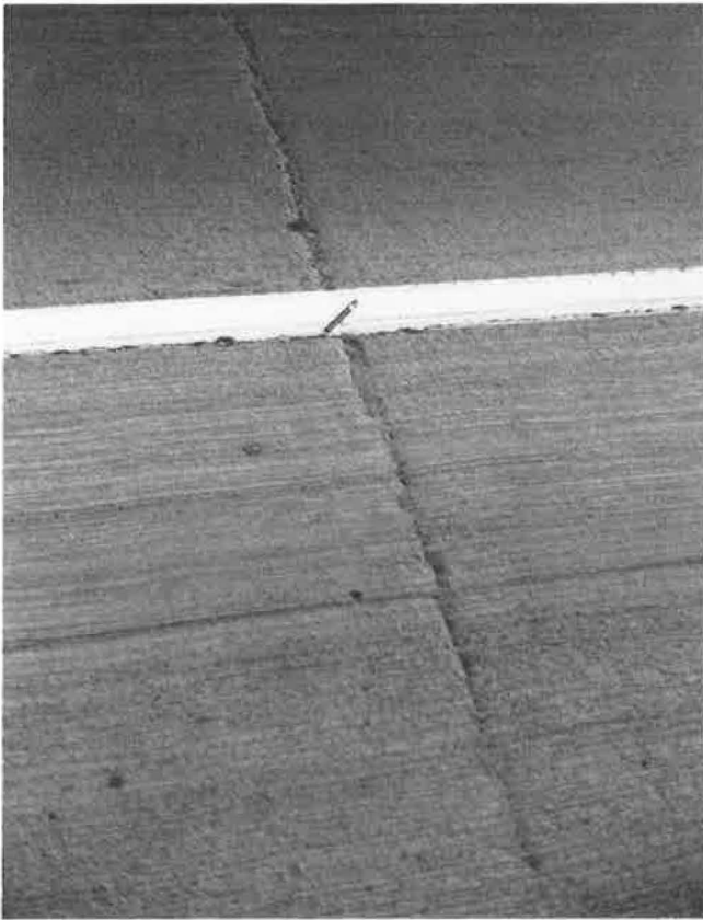
FIGURE 14 Depression caused when paving train stopped.
