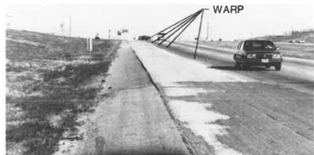
FIGURE 1 Observed pavement warp, Westbound, I-635 near MacArthur Blvd., Irving, Texas. Design section shown in Figure 4.
