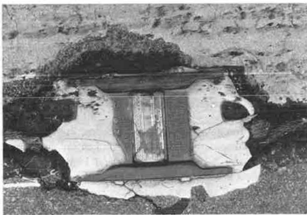
FIGURE 3 Cracked reflector with top and side delamination.
