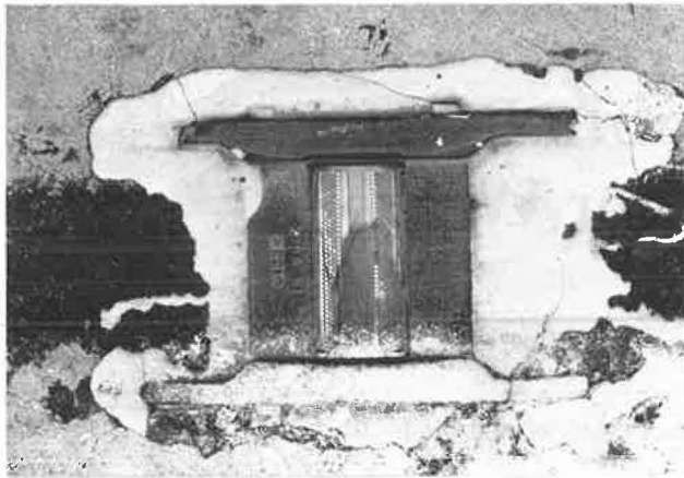
FIGURE 2 Cracked reflector with top delamination.
