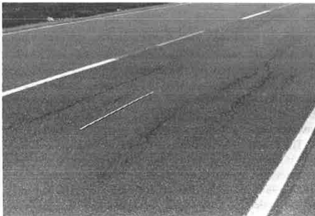
FIGURE 9 Longitudinal surface cracking.
