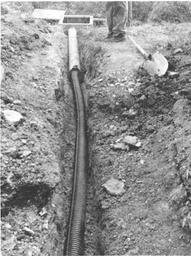
FIGURE 16 New outlet pipe.
