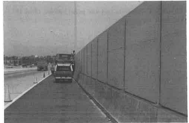
FIGURE 9 Cameo double-layered aluminum barrier along I-280 in Harrison, New Jersey.
