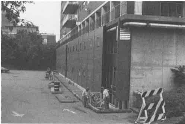
FIGURE 10 Modular sound wall affixed to exterior of Rutgers University building.
