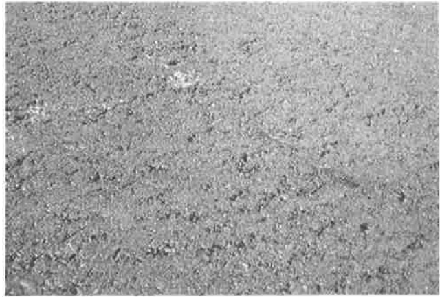
FIGURE 12 Surface cracks of steel-compacted asphalt (field trial in Egypt).
