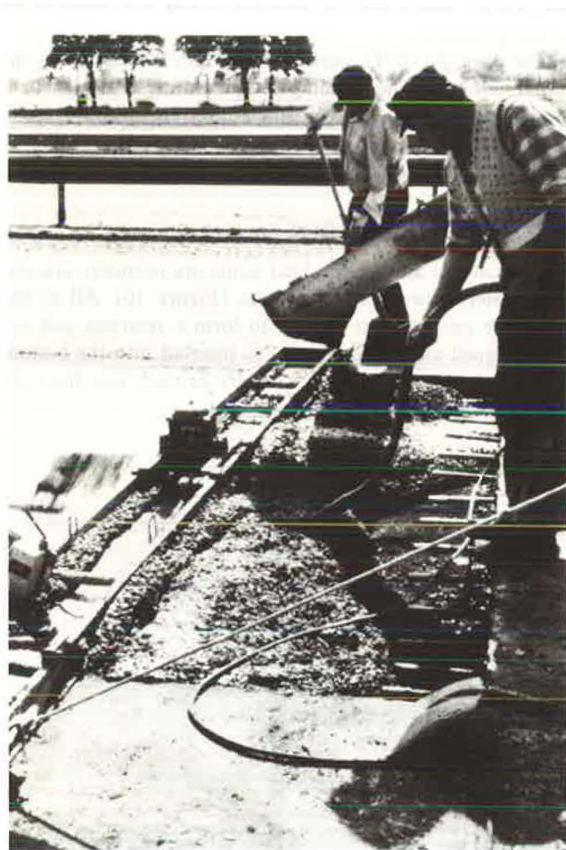
FIGURE 12 Paving and compacting of high-early strength concrete for 1-day reconstruction of concrete slabs (fast track concrete paving).
