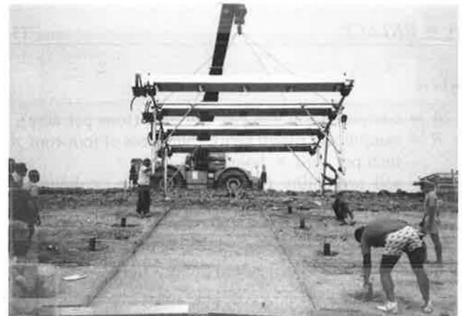
FIGURE 3 Crane lifting rainfall simulator from highway shoulder to test plot on 3 to 1 slope.
