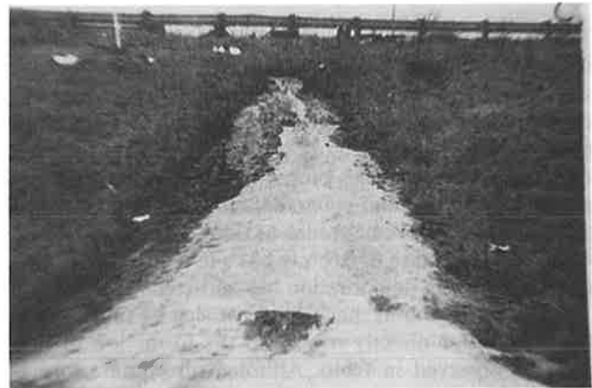
FIGURE 3 Tufa precipitate flume on fill slope.
