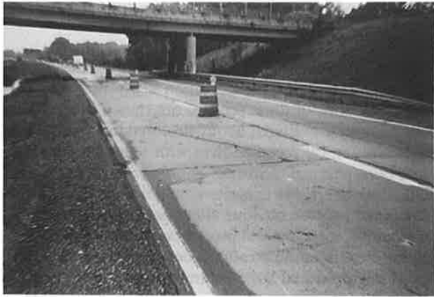
FIGURE 4 Deteriorated pavement section.
