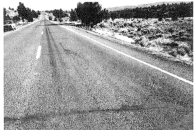
FIGURE 9 Typical cracking—transverse, test segments 9 and 10, 0.30 and 0.50 ft conventional DGAC (age 48 months).
