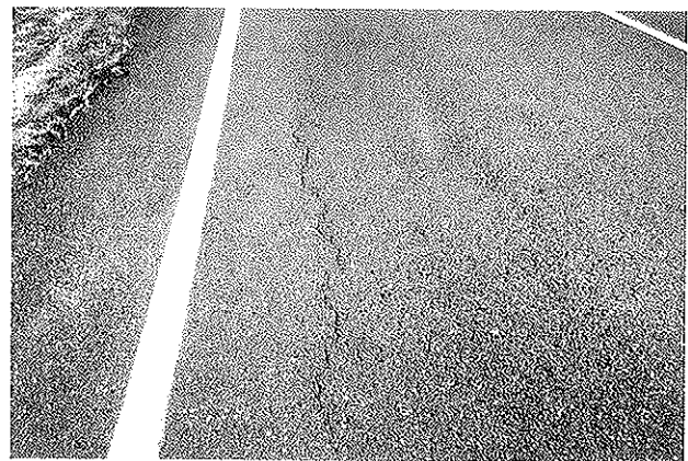
FIGURE 4 Typical Cracking—longitudinal, test segment 2, 0.15 ft ARS DGAC on SAMI (age 48 months).
