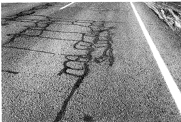
FIGURE 7 Typical cracking, test segments 7 and 8, 0.15 and 0.20 ft conventional DGAC (age 48 months).
