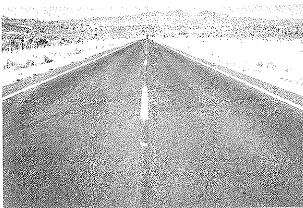
FIGURE 14 Typical "overall" view, ARS DGAC (age 48 months).
